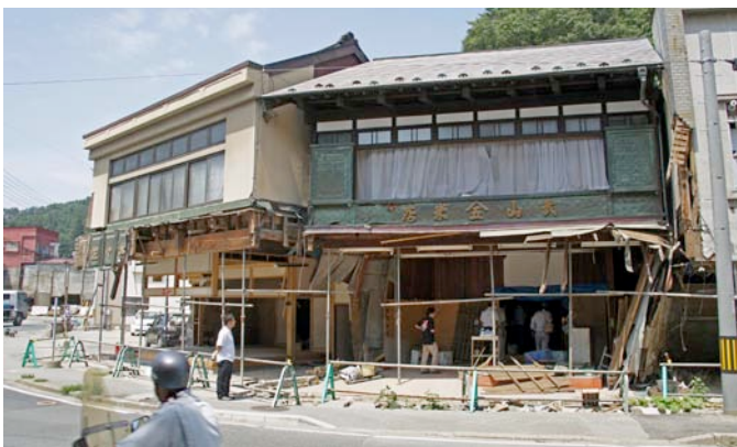
EARTHQUAKE DAMAGE, JAPAN
